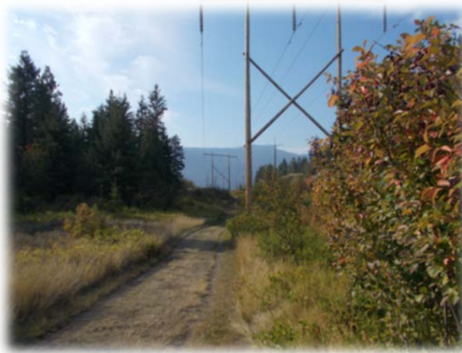
Plate 2: The Fortis BC transmission line travelling through the core area of the park (Rattlesnake Hill).
