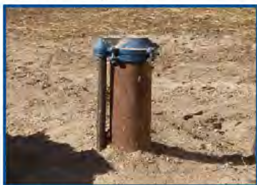
Figure 6. Well fitted with pitless adapter, cap has space for wiring
