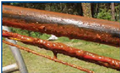
Figure 3. Biofilm on well wiring
