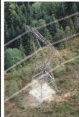
BC Hydro 500 KV transmission line
