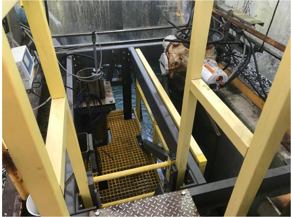
Photo 3: Sampling facility and : main effluent gate valve
