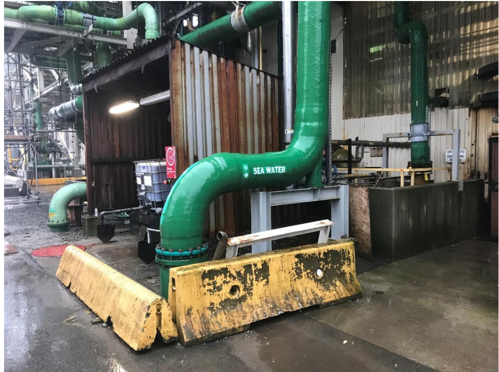
Photo 1: The sea water pumped into the Site to be used as cooling water is transported around the Site in green pipes.
