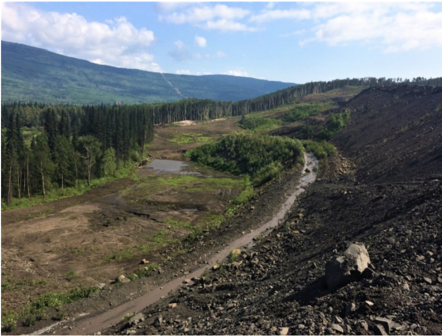
Photo 2 - Proposed 4N1 Pit haul road area looking east. The existing east/west diversion ditch conveys water from the pit the North Pond.
