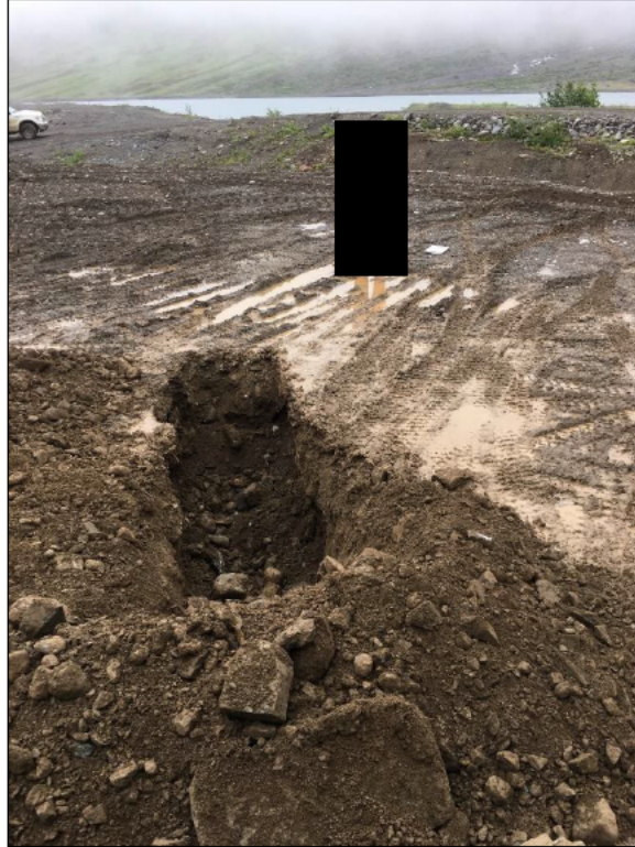
Photo 4.1-12: Test Pit - Cell 2 location to ensure adequate depth of levelling base course.
