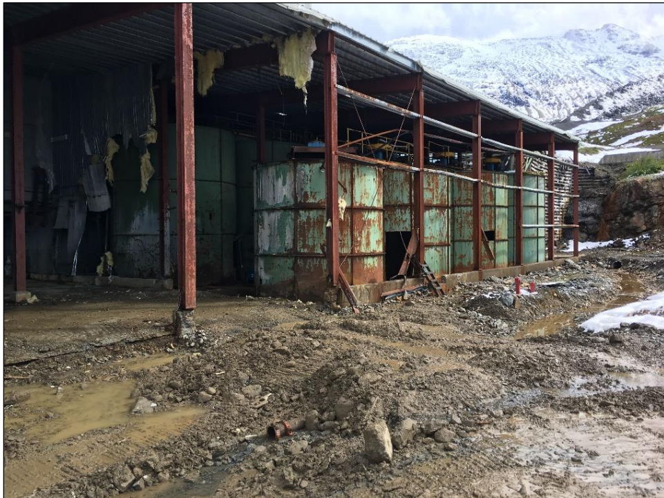
Photo 4.1-5: Cyanide tanks within Mill Building.
