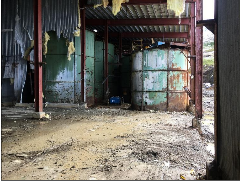
Photo 4.1-4: Cyanide tanks within Mill Building.
