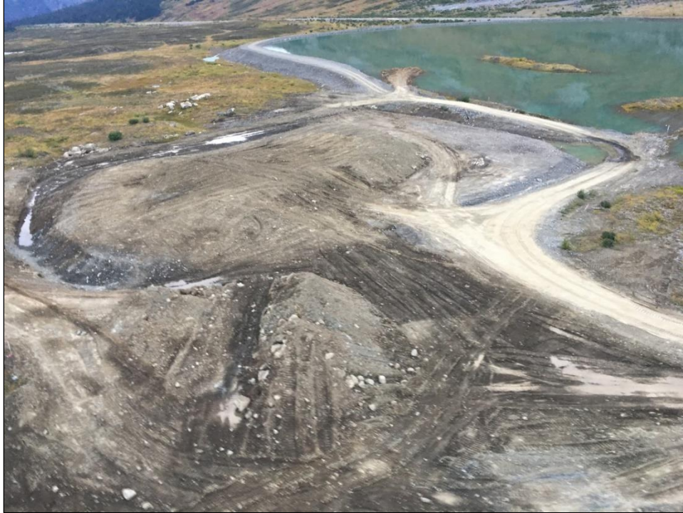
Photo 4.1-14: Main Landfill Area - Waste material covered with mineral soils to a minimum depth of 300 mm.
