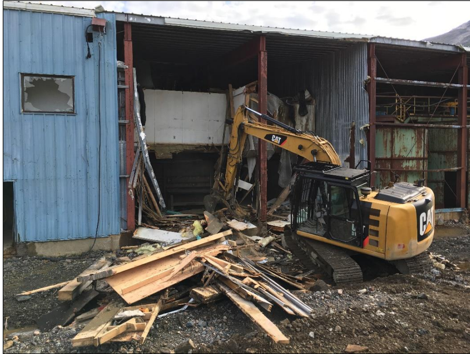
Photo 4.1-1: Mill Building - Wooden construction waste piled and burned.
