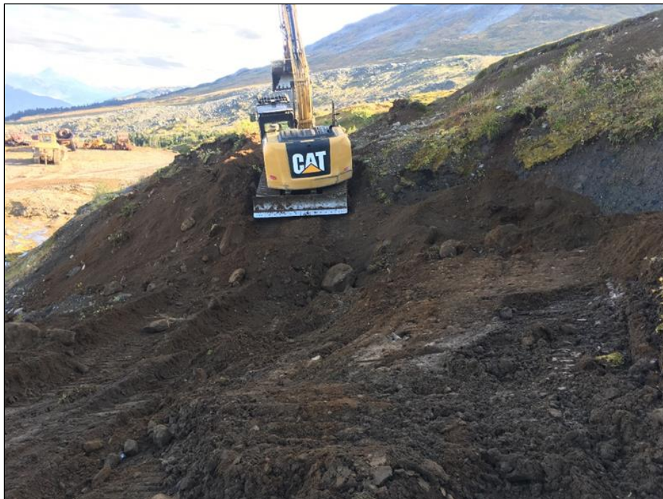
Photo 4.1-15: Portal 11 - Additional Grading Required above Portal Entrance.
