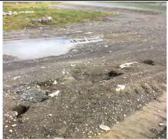
Photo 3: Vantage point photo along northern edge of the Main Landfill. Minor erosion observed along north slope. Ponding of water was observed in the northern access road..
