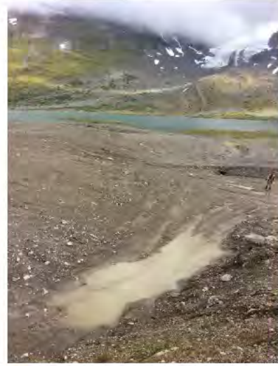
Photo 13: Vantage point photo of southwestern edge of Main Landfill looking east towards the culvert. Ponding water was observed in this area.
