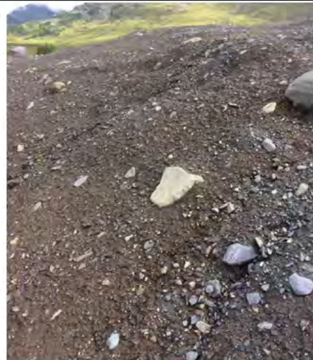
Photo 7: Vantage point photo along western slope of the Main Landfill looking northeast. Minor rill erosion was noted.
