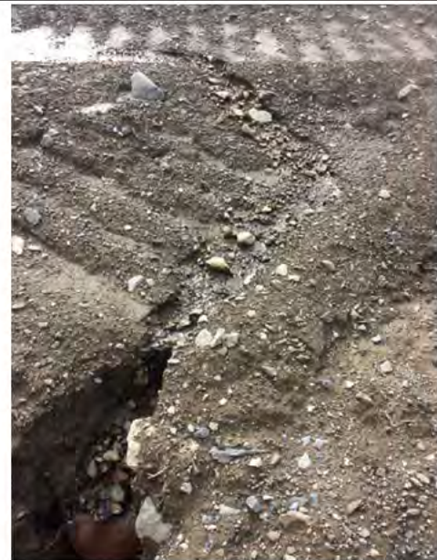
Photo 5: Close up of erosion noted on north slope including some exposed metal.
