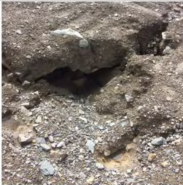
Photo 4: Close up of erosion noted on north slope including some exposed metal.
