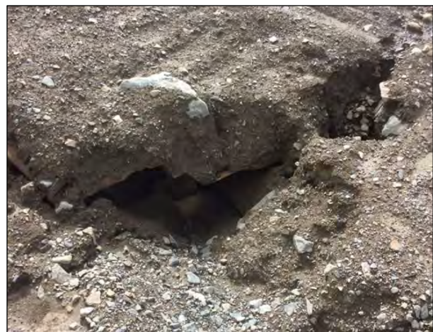
Photo 8-4: Close up of erosion noted on north slope including some exposed metal.
