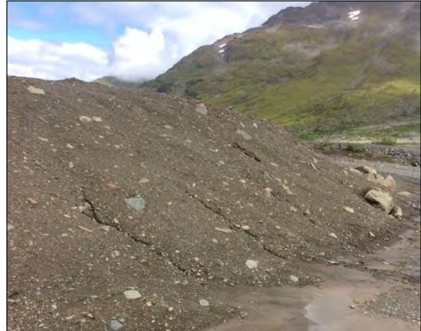
Photo 8-2: Vantage point photo of south edge of Main Landfill looking northeast. Minor erosion was noted on south slope of Main Landfill.
