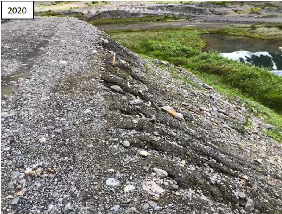
Photo I-21 South Corner Rill Erosion (G-5)
