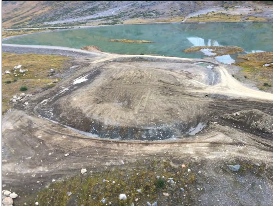
Photo 2.2-1: Main Landfill - Cell 1 and 2 covered, recontoured and compacted to drain to the TSF (2019).
