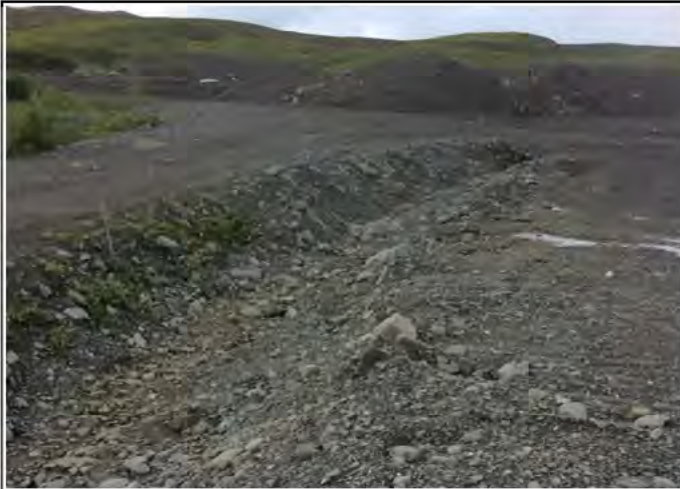
Photo 2: Vantage point photo of southeast Corner of Cell-2 looking northwest. South ditch east of culvert observed to be dry.
