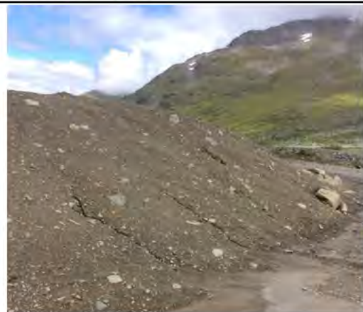
Photo 11: Vantage point photo of south edge of Main Landfill looking northeast. Minor erosion was noted on south slope of Main Landfill.
