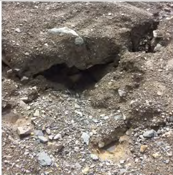
Photo 4: Close up of erosion noted on north slope including some exposed metal.
