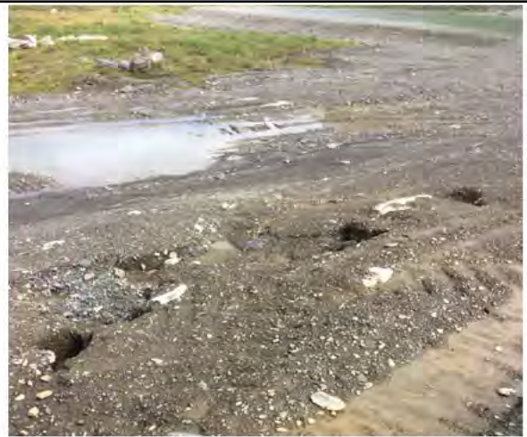
Photo 3: Vantage point photo along northern edge of the Main Landfill. Minor erosion observed along north slope. Ponding of water was observed in the northern access road..
