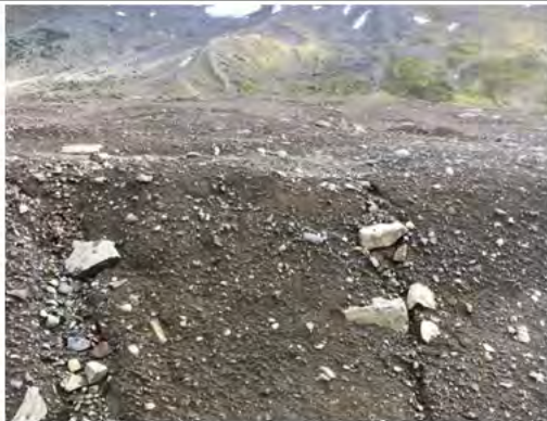
Photo 8: Vantage point photo along western slope of the Main Landfill looking east. Minor rill erosion was noted.
