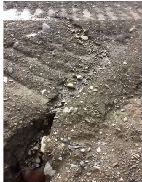
Photo 5: Close up of erosion noted on north slope including some exposed metal.
