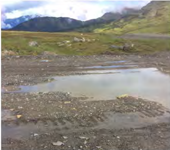
Photo 6: Vantage point photo along northern access road of the Main Landfill. Ponding of water was observed in this area.
