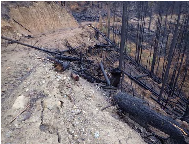
Photo 24. Firebreak road branching off Road R06128-191. Oversteeped fillslope with tension cracking presents landslide hazard above Slim Creek FSR. Permanent deactivation required.
