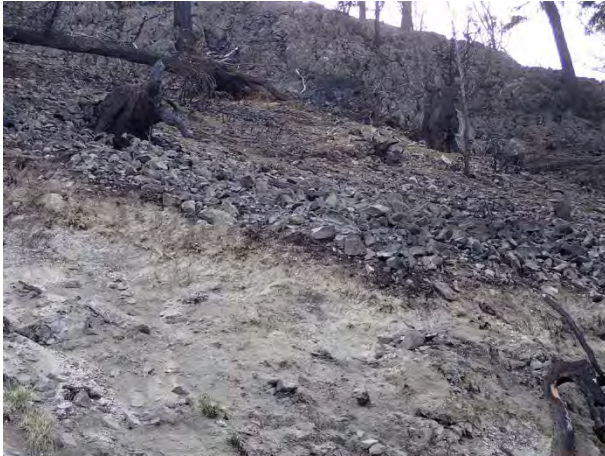
Photo 5. Rockfall fragments below rock outcrop form veneer covering tephra visible in road cut along Slim FSR.
