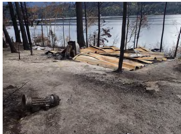
Photo 10. Burnt structure in area outside fire tornado. Roofing falls directly down on foundation.
