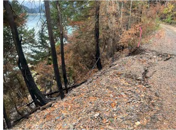
Photo 21. WP DK7. Burnt wood creating driving hazard.
