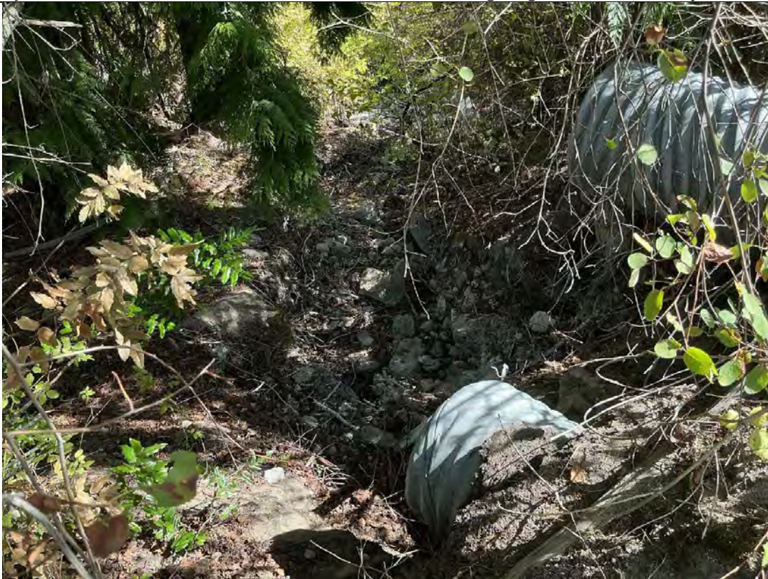
Photo 6: Quilpituk Creek culvert outlets (500 mm and 600 mm diameter) at Westside Road, view downstream. Note the deep channel scour indicative of high flow conditions. Only a small trickle (<0.5 litres/sec) of water was flowing at the time of the field assessment.
