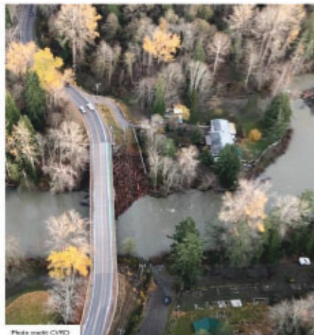
Photo 11: Large woody debris on right abutment of Chemainus Road Bridge after November 2021 flood which has since been removed
