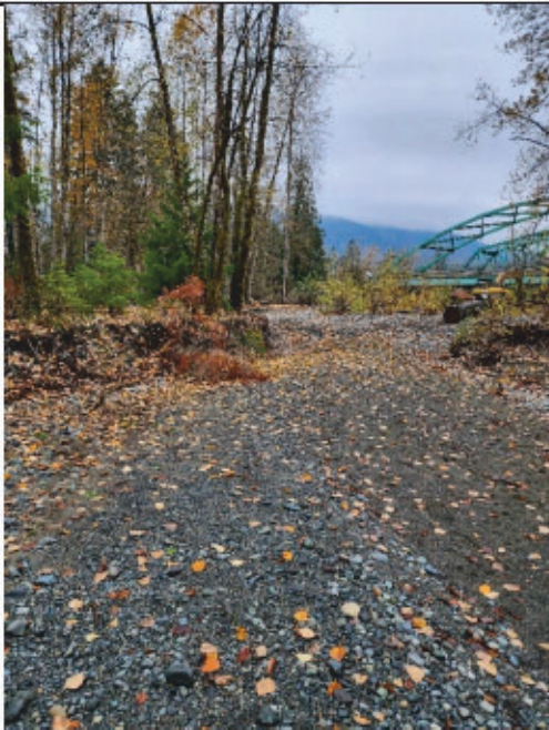
Photo 1: Area of concern, looking upstream, the left bank is lower in elevation than the new channel alignment. Possible over-topping point of new channel.
