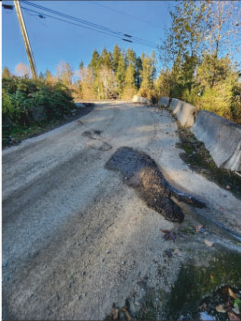
Photo 1: Drainage curb, destroyed by dump trucks, to be reinstated.
