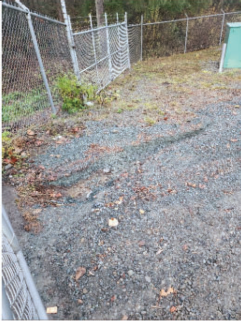
Photo 1: Deep scouring just below asphalt curb. Not sure if it is from a vehicle tire or water.
