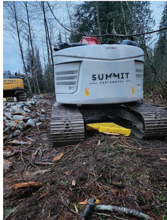
PHOTO #4 – Spill tray under parked 245 Excavator
