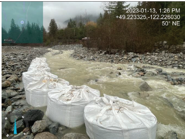
Photo 16. Elevated background turbidity at the upstream extent of the site. SEI notes that the origin of the observed turbidity was from outside of site (Jan 13, 2023).
