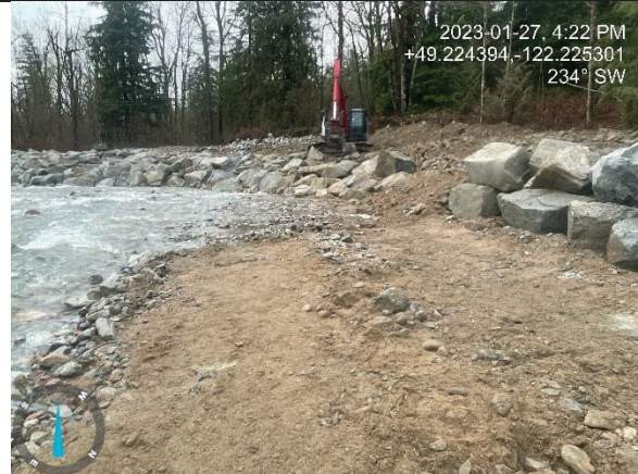
Photo 13. Southwest-facing view of deflection gravel berm bags removed. Right creek flow 50%, left creek flow 35%, middle creek flow 15%. (Jan. 27, 2023).
