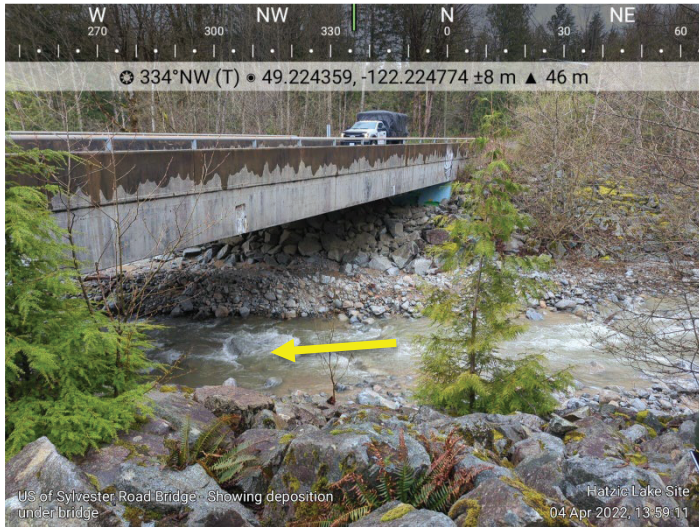
Deposition in Pattison Creek below Sylvester Road Bridge
