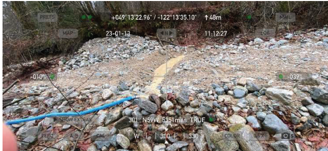
Figure -9 Looking westerly at pumped out excess water settlement
