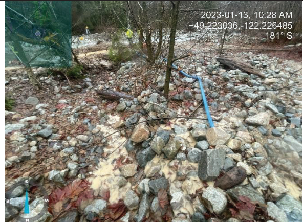
Photo 14. Outlet of the of the 2 inch hose; turbid water was pumped to ground away from Pattison Creek for infiltration (Jan. 13, 2023).
