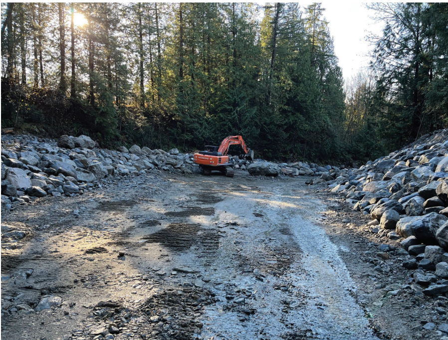
Photo 3. Jakes armouring banks downstream of the debris jam.
