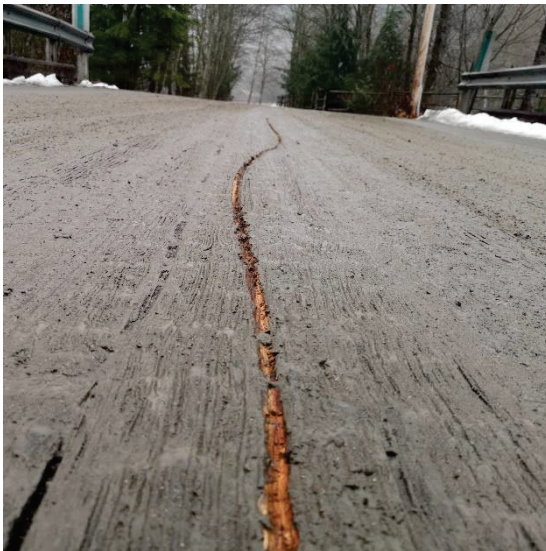
Figure 2-3 Gouge in Bridge Surface
