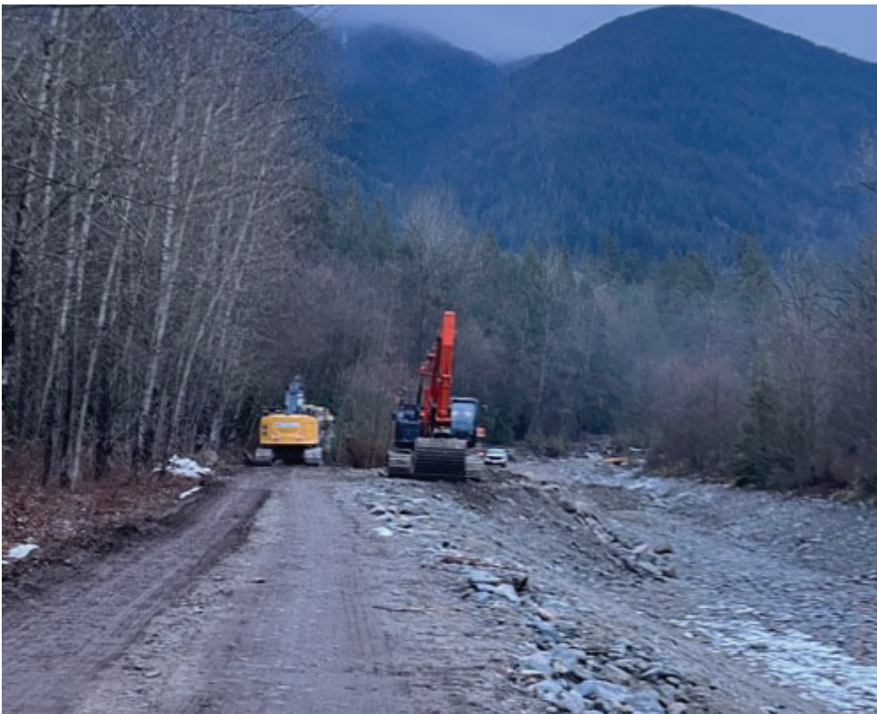
Photo 3. Machinery parked on top of bank along dike road overnight.
