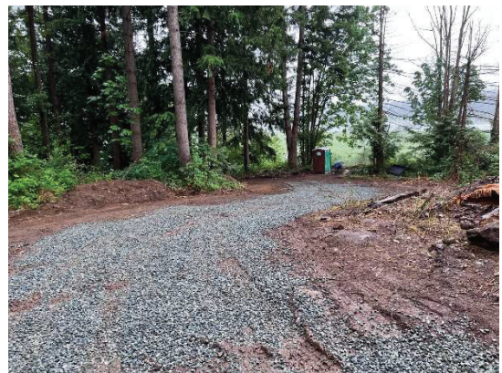
Figure 4 Gravel Spread on Steep Slope
