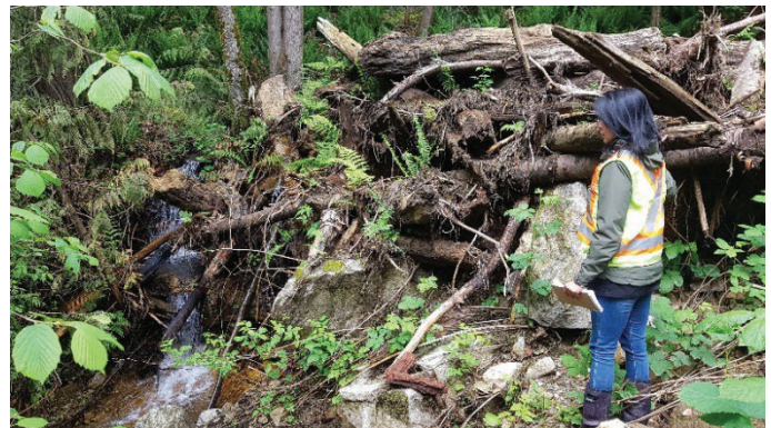
Davies Creek – Upstream Log Jam (Looking Upstream)
