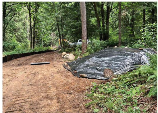
Figure 2 Stockpile Covered with Poly Sheeting
