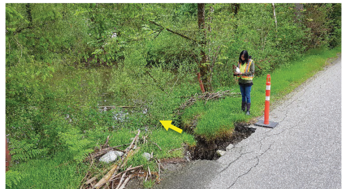
Damage to north Shoulder of Hartley Road 100 m west of Hartley Road Bridge Looking Southwest
