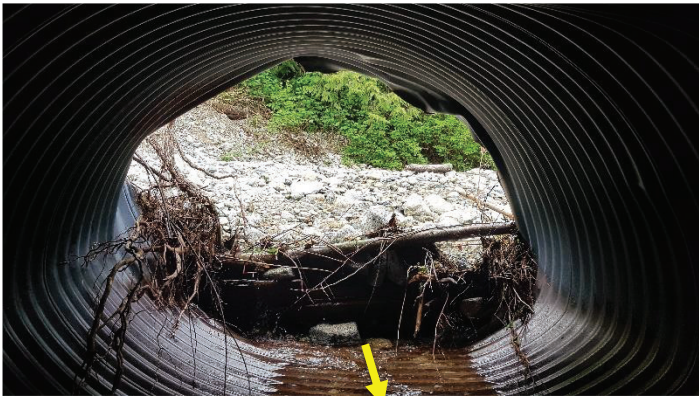
Upstream blockage of northern MacNab Creek culvert at Sylvester Road
