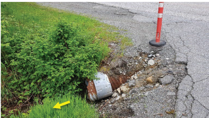
Erosion at Sylvester Road and Hartley Road intersection (west shoulder) Looking Northeast
