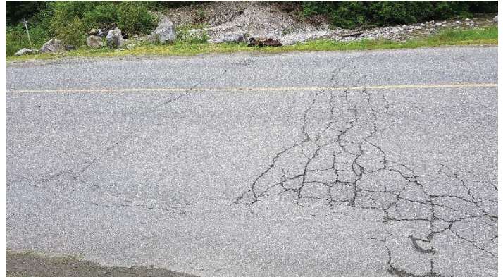
Pavement cracking on Sylvester Road aligned with both culverts.
