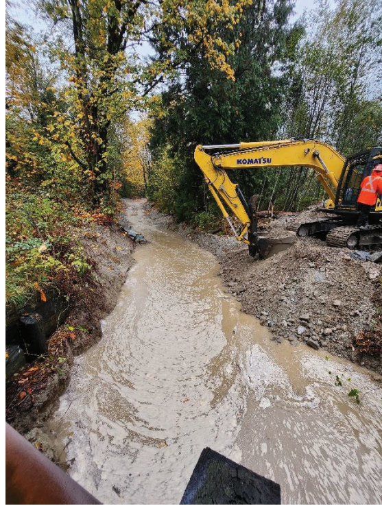
Figure 6 - Poor visibility preventing rip-rap placement
