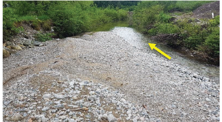
Deposition in MacNab Creek downstream of Sylvester Road culverts
