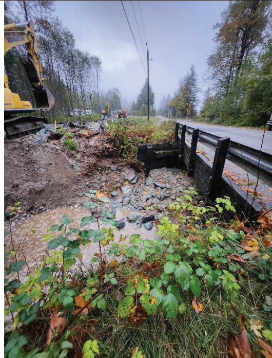
Figure 2 - Photo showing disconnection of water to below Sylvester Rd Bridge
