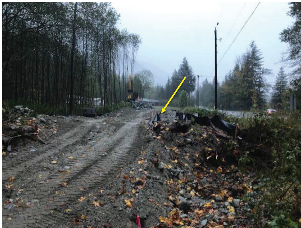
Photo 3: Silt fencing requiring repair.
