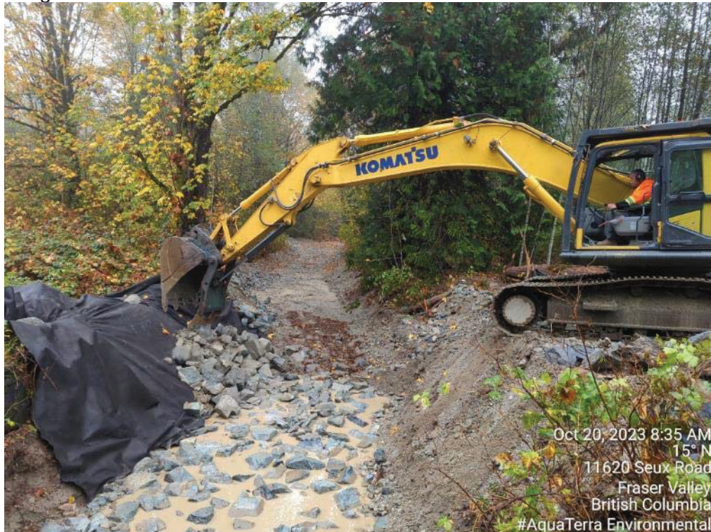
Photo 5: Riprap covering geotextile material with large pool of standing water observed in the foreground.
