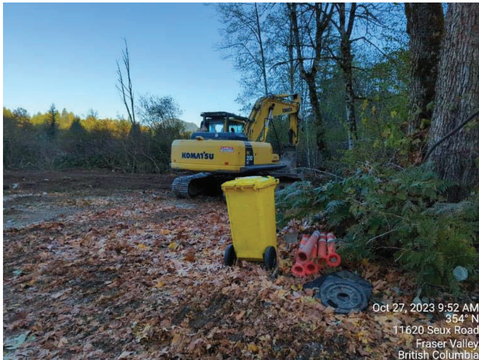
Photo 16: One (1) large and fully stocked spill kit observed in staging area.
