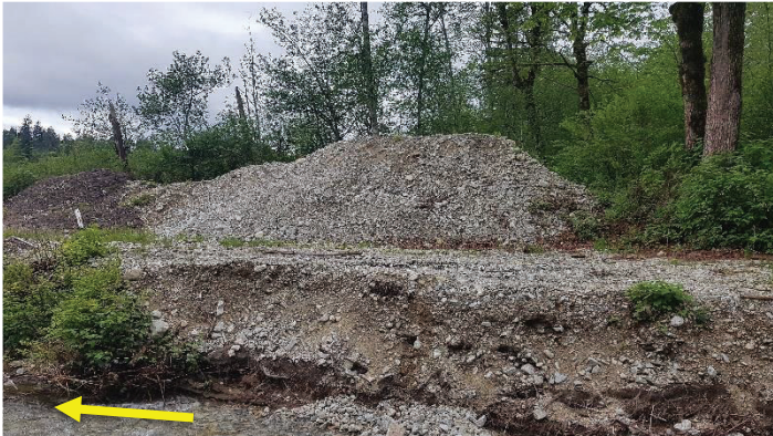
Excavated Materials downstream of Sylvester Road culverts
