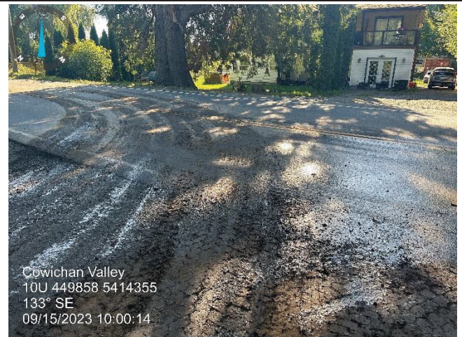
Photo 6: Track out on Chemainus Road after water application
