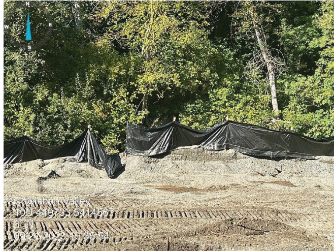
Photo 1: Damaged section of amphibian exclusion fencing
