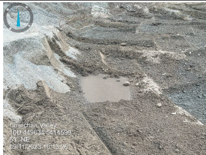
Photo 3: Small groundwater infiltration
