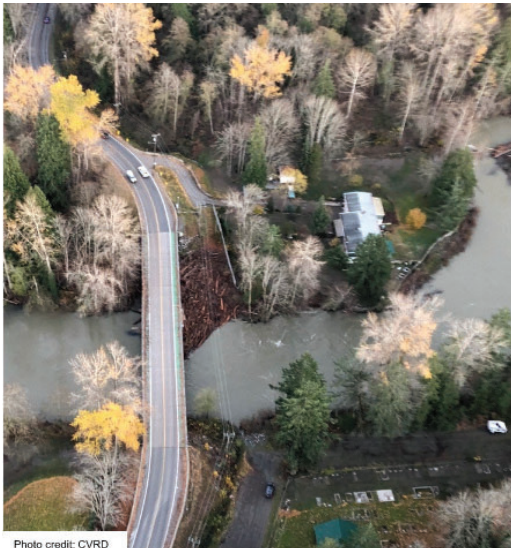
Photo 15: Large woody debris on right abutment of Chemainus Road Bridge after November 2021 flood which has since been removed (Source: NHC 2022)
