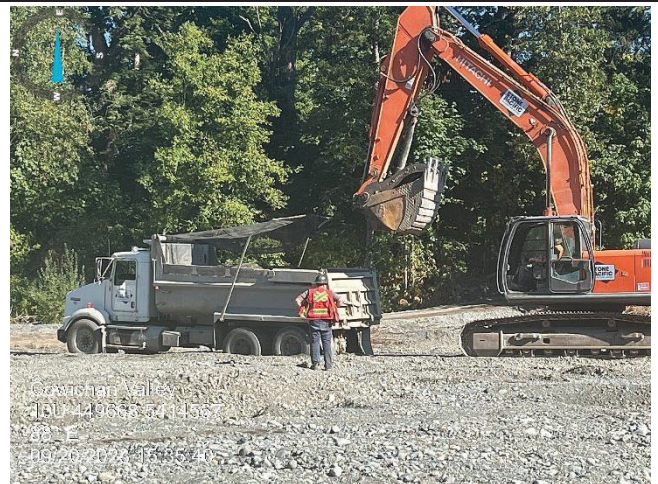
Photo 4: Dump truck stuck on gravel bar
