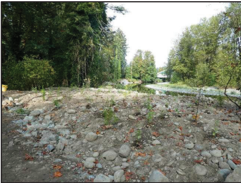
THE AREA IMMEDIATELY ABOVE WEIR 6 AFTER BEING REPLANTED.
