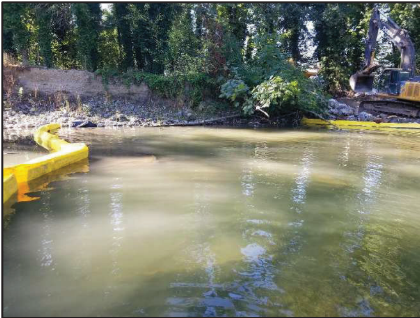
TURBID WATER THAT SEEPED OUT OF THE ISOLATED AREA FROM UNDER THE SILT CURTAIN. TURBID WATER WAS CONTAINED IN THE IMMEDIATE AREA AND DID NOT REACH THE LOWER WATER QUALITY SITE.
