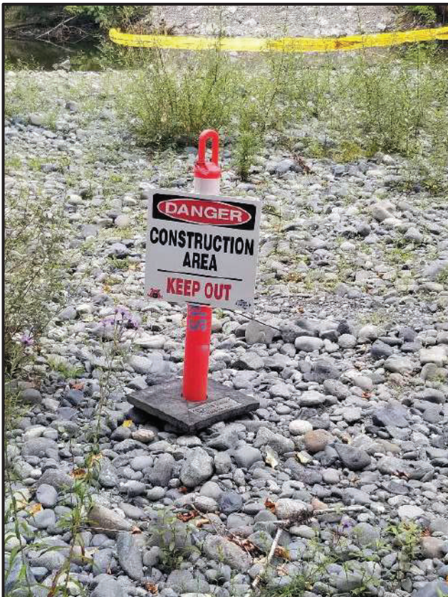
WARNING SIGNAGE POSTED ON THE LEFT BANK OF THE CHEMAINUS RIVER OPPOSITE THE MAIN WORK AREA. SIGNS WERE PLACED AT THE MOST COMMON PEDESTRIAN ACCESS POINTS.
