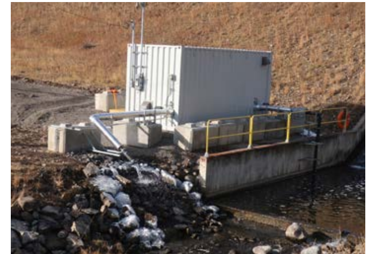
Figure c. Calcite antiscalant dosing skid on lower Greenhills Creek.
